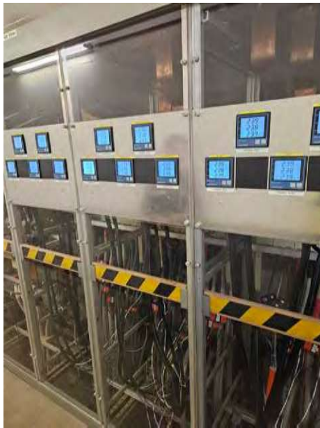
Picture 3 – Measuring devices in one of our electrical energy distribution cabinets
