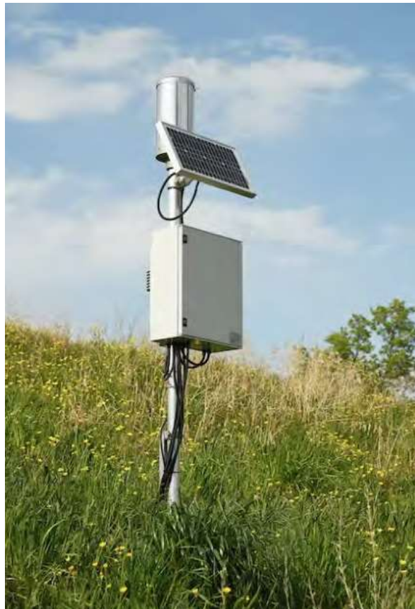
Picture 2 - One of three installed temperature measuring stations
